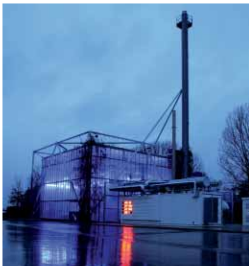
Co-generator powered by renewable raw materials
