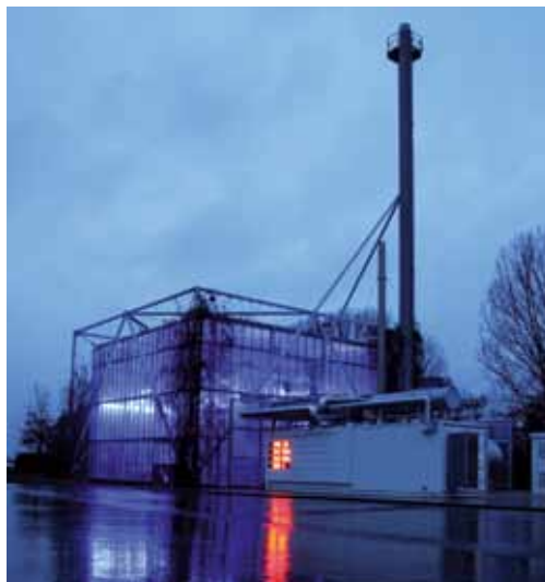
Co-generator powered by renewable raw materials
