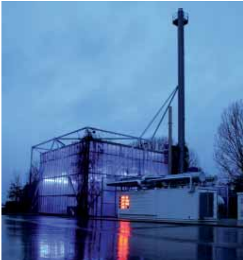
Co-generator powered by renewable raw materials
